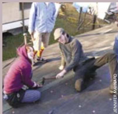
Alison Holt '08 and Jake Blumgart '08 repair the roof of a house in Bogalusa, La., during a January work trip.
