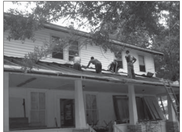
Students help replace the roof of the Quaker Lodge during a fall work trip to Choctaw Friends Center. Find out more on page 7.
